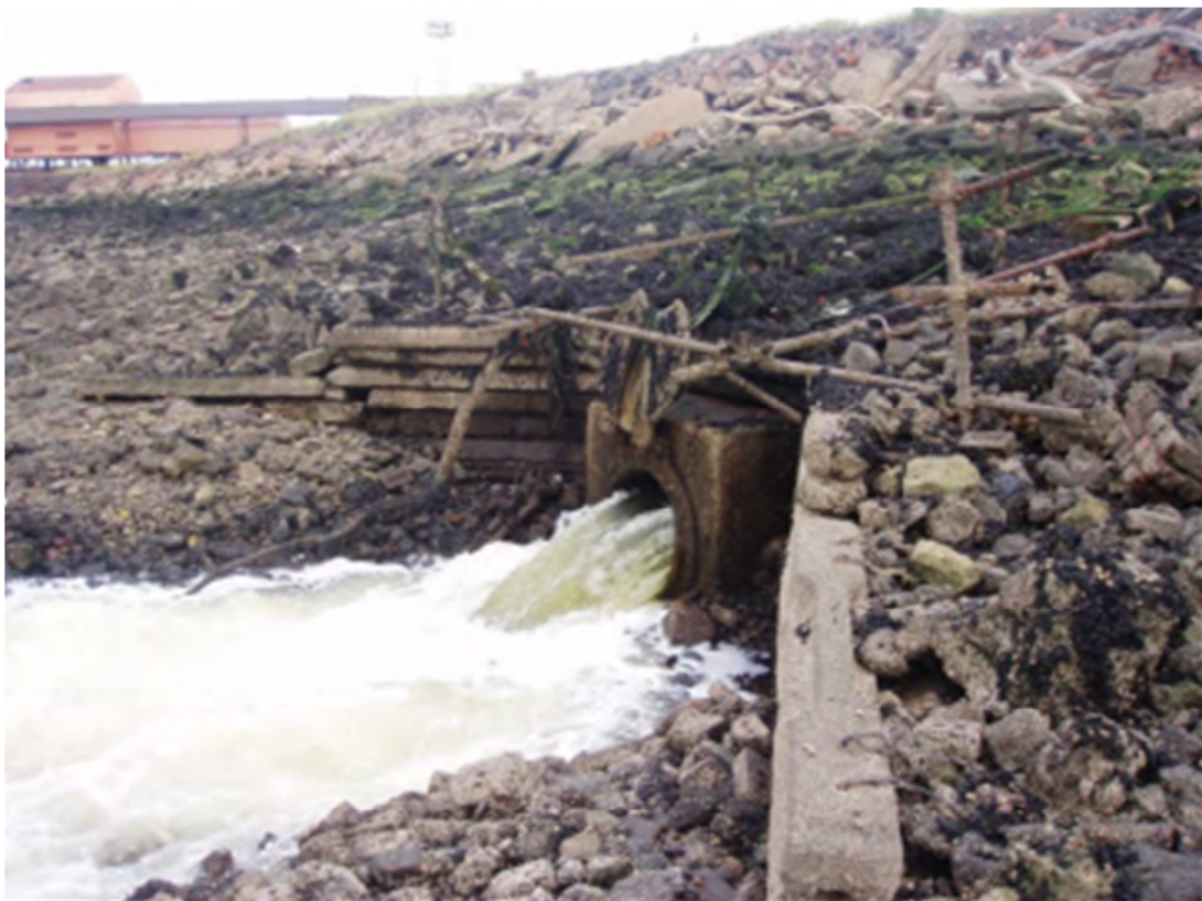
Figure 5.9 Pipe connecting Bran Sands Lagoon to the Tees estuary
